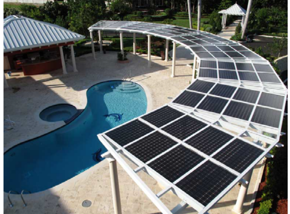
Example of solar panel installation on pergola type feature
