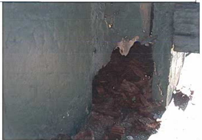
Photo #4: View of base of rotted post.
